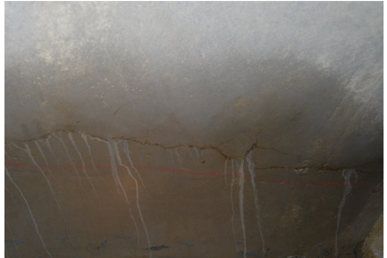
Fig. 3: A typical crack in the pipe wall
