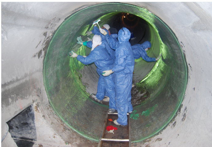
Fig. 5: Installation of FRP sheets on the interior surface of the pipe. An access point is visible at the lower left
