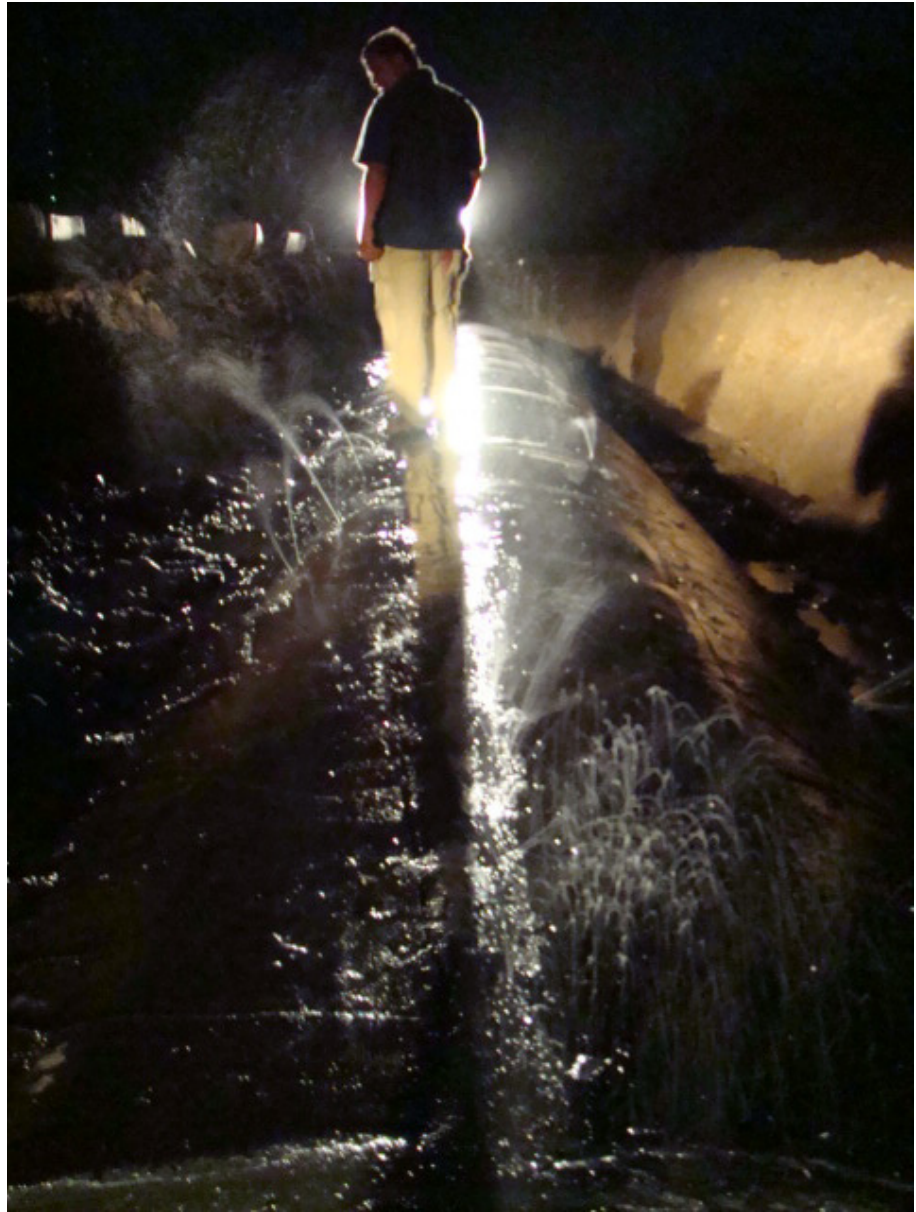
Fig. 2: After conventional crack sealing, the penstock failed to pass a second pressure test.
